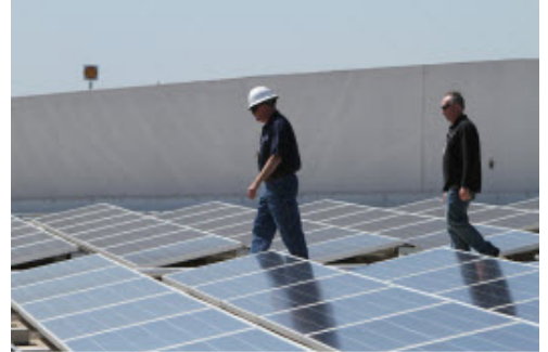
Assurant Specialty Property's new solar panels
