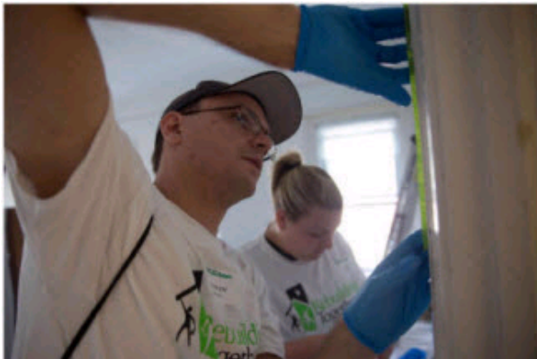
Assurant volunteers apply a fresh coat of paint to a home on Dare Court on June 6, 2013 in Gerritsen Beach, Brooklyn
